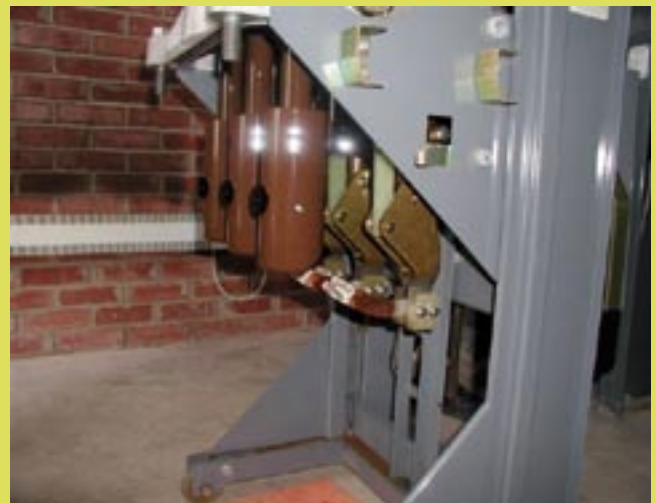
An 11kV circuit breaker which has been isolated for maintenance.
