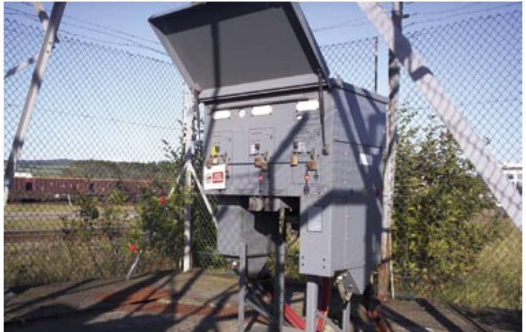
An 11kV ring main unit at Tyne Yard.
